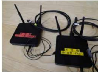
1 unit Used to send projection data from inside the hall to the control room Multipurpose hall
