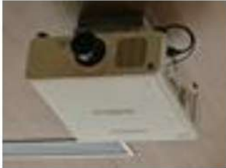
1 unit/Panasonic/PT- RZ970J/10,000lm Multipurpose hall
